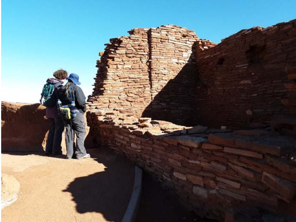
Two RCC Field Trippers Examining Wall Masonry Construction at Backside of Wupatki
