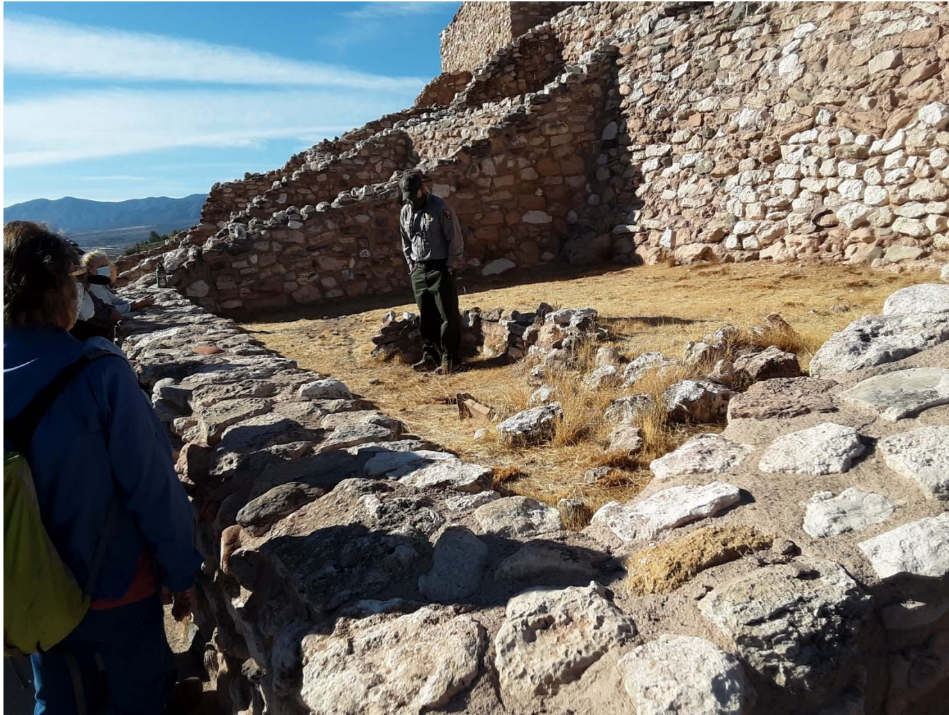
National Park Service Archaeologist Matt Guebard standing in a large subfloor structure left exposed by the excavators. The wall behind him had partially collapsed many years ago due to water pressure not relieved by proper drainage. The upper portion was reconstructed from the original stones, revealed by the different color and pattern of the upper portion.
