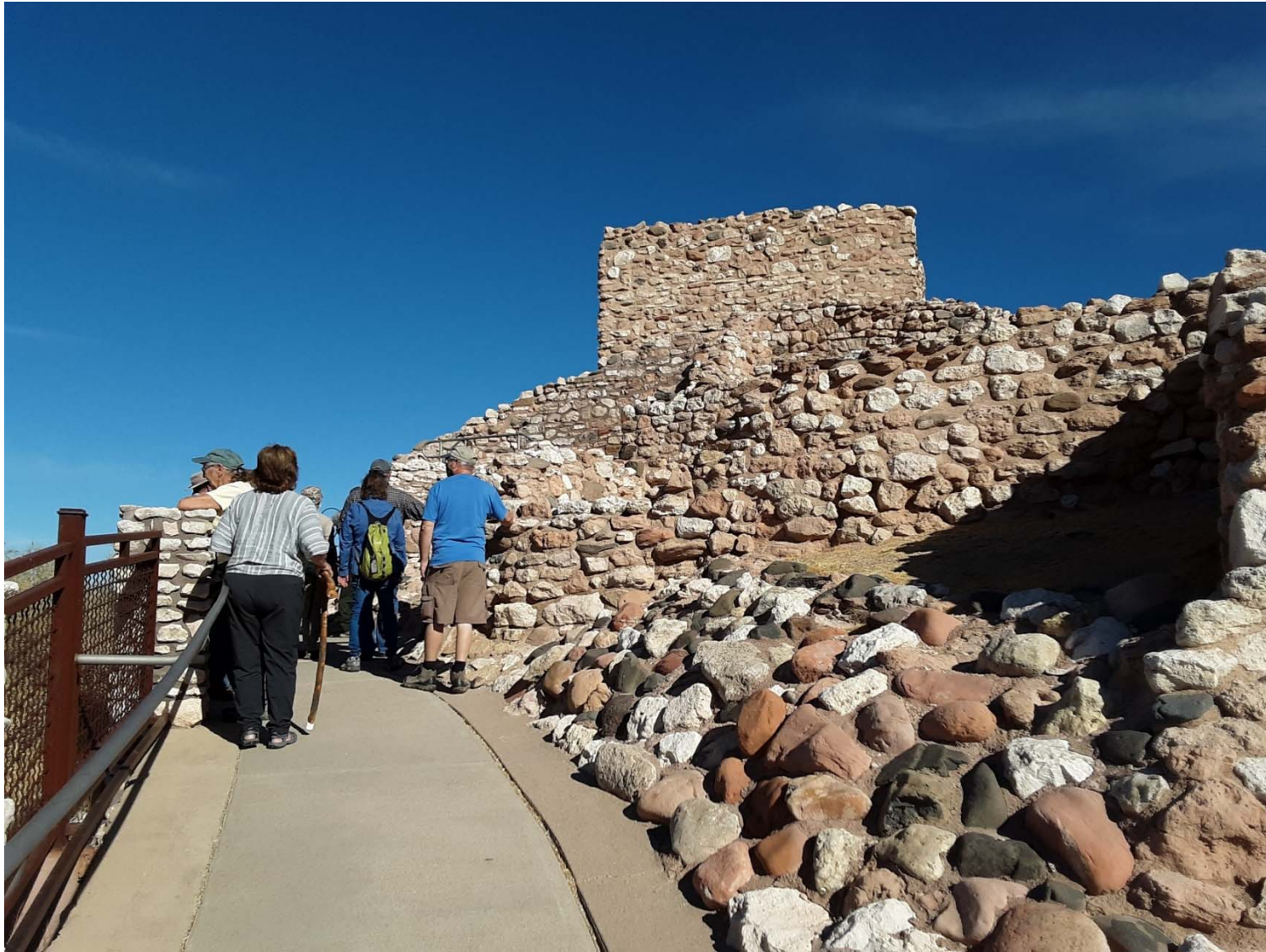
Highest point of Tuzigoot Pueblo. Here there is a wall with original plastering on it, not currently available for viewing, due to roof safety issues.
