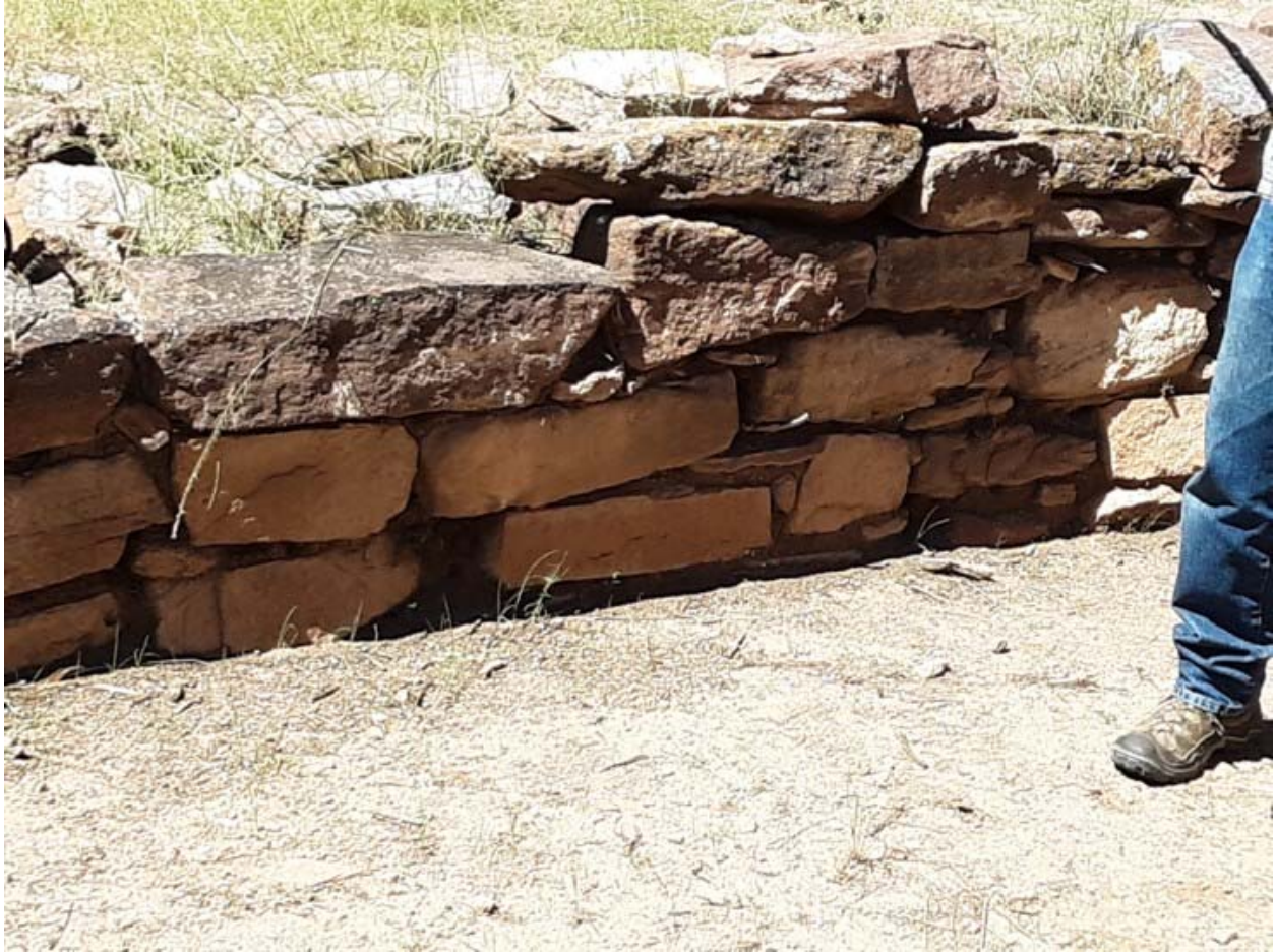
Coursed large stone masonry of Room 8 along Courtyard Feature 29 in front of it. At least some of the stones appear to have been “dressed” before use, not just taken and used as found.
