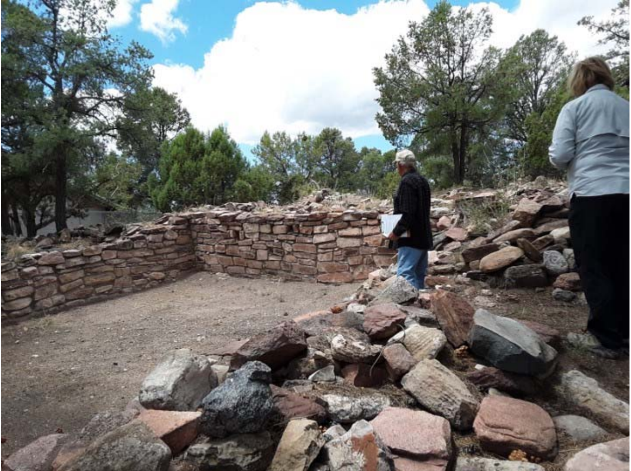
The Wall in Back is the one which Collapsed and was Restored
