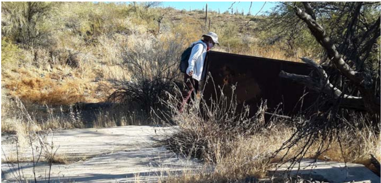
Rusted Rectangular Steel Tank and Concrete Slab
